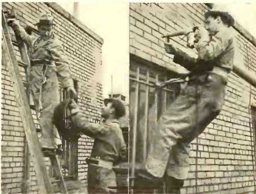
Installations on apartment houses require a well-trained serviceman. Servicemen are shown installing a Taco master aerial system. Performance and reliability are paramount in this type of work.
